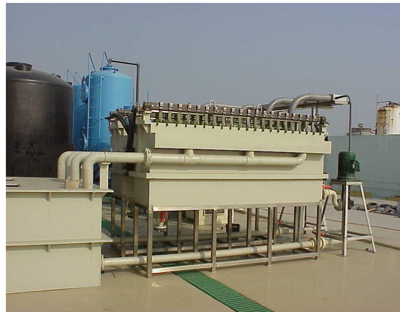
The full scale ion exchange and ER system for copper removal. (WUS Printed Circuit, Taiwan)
